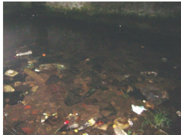
Picture 8: Basement of the School # 3 in Chkhorotsku
